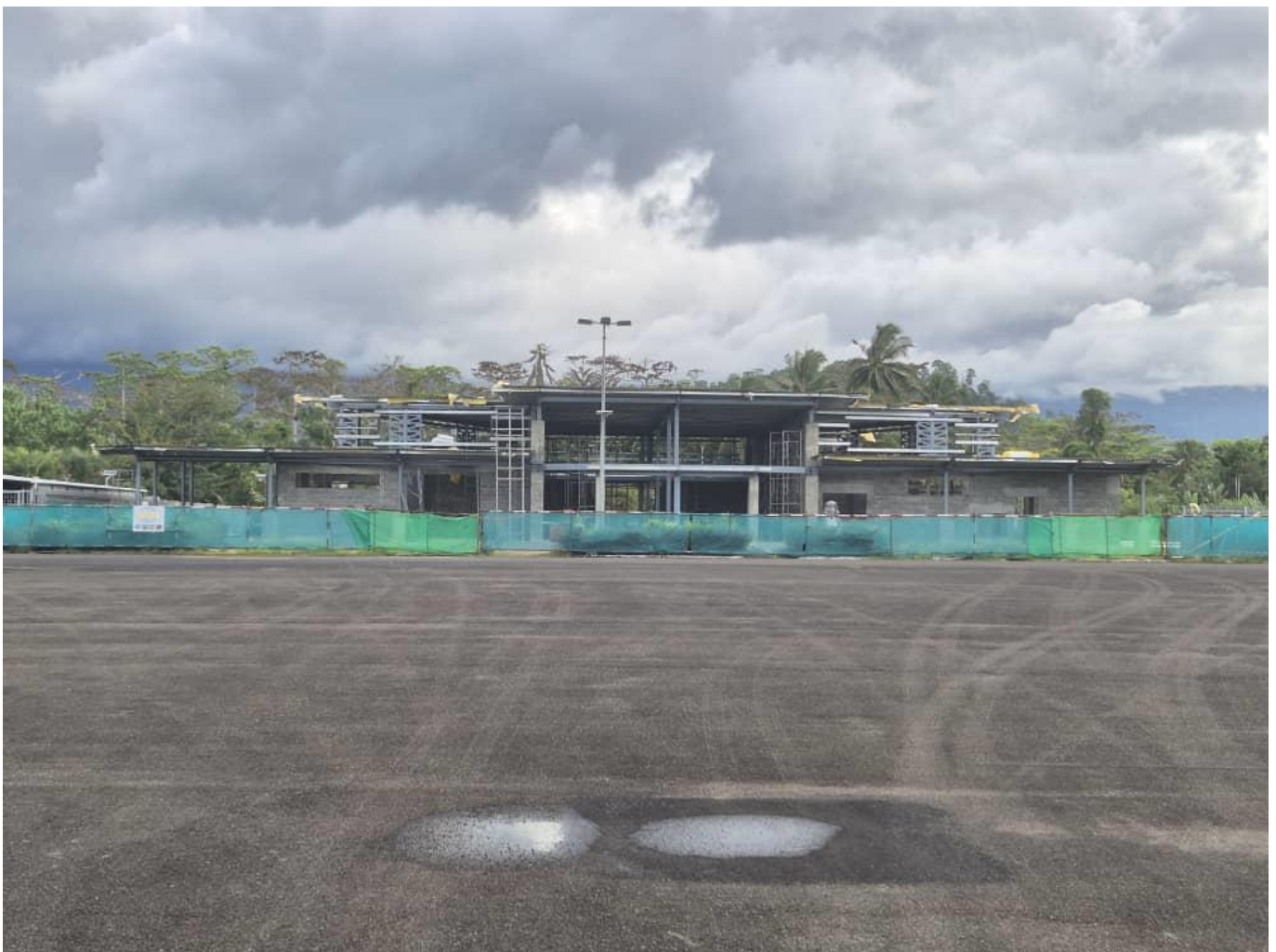
Caption 3: Construction of the new terminal building at Kieta Airport in progress.
