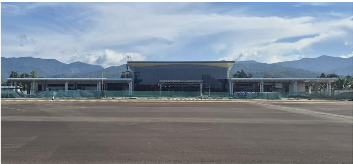
Caption 3: Construction of the new terminal building in progress at Gurney Airport (Airside).
