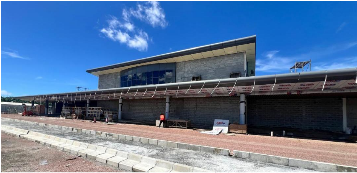
Caption 4: Construction of the new carpark and terminal building in progress at Gurney Airport (Landside).
